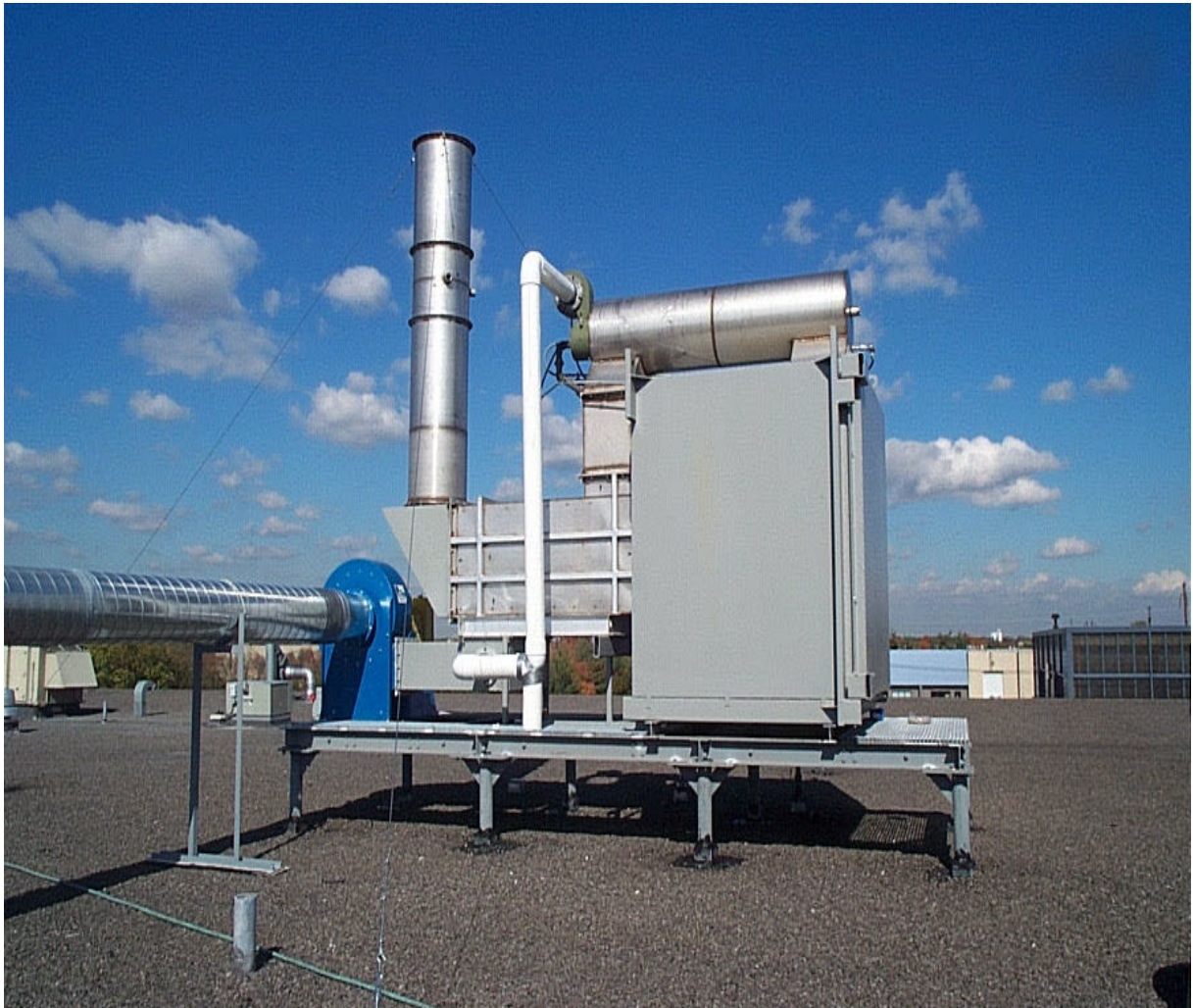
8,000 SCFM Catalytic Oxidizer with Preheat Exchanger
